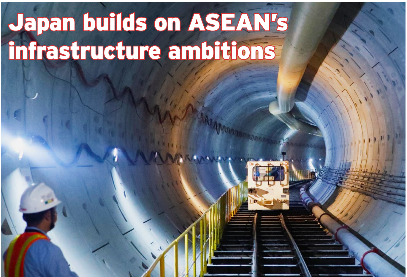
A worker stands in a tunnel of the Jakarta Mass Rapid Transit project funded by the Japan International Cooperation Agency (September 2022).
